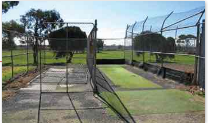
Infill previous safety and maintenance hazard area with compacted granitic sand and 25mm pile synthetic grass.
