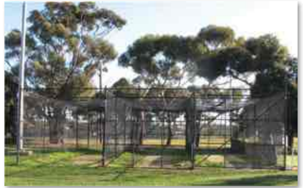
Example of poor quality and unsafe infill materials Image courtesy of insideEDGE Sport and Leisure Planning
