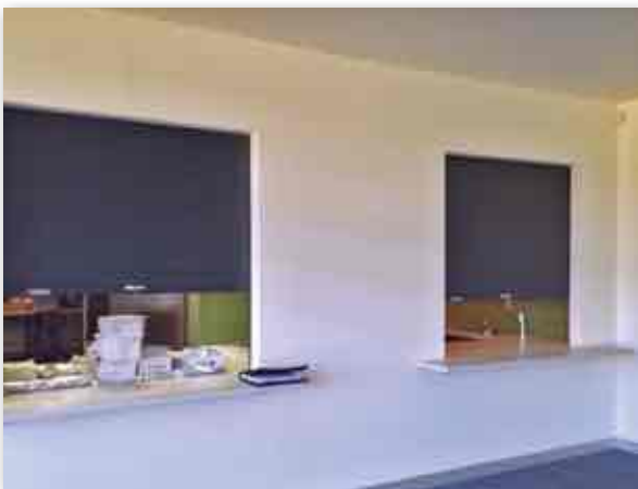
Example of internal multi-purpose room and kitchen servery Image courtesy of JMA Architects
