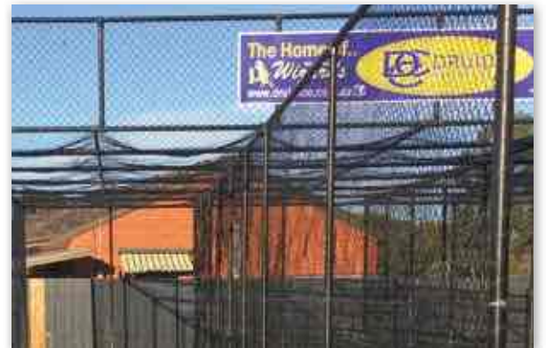
Example of damage to a flat roof net design Image courtesy of insideEDGE Sport and Leisure Planning
