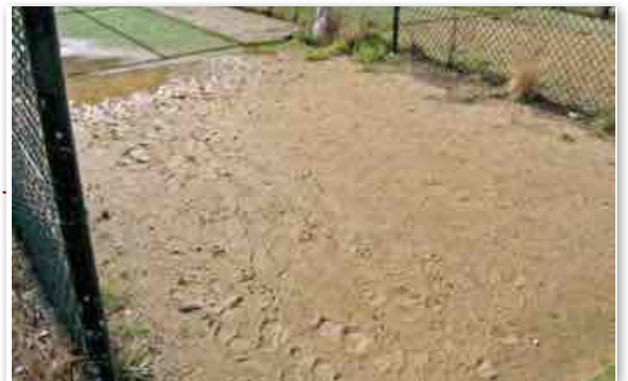
Join existing batting and bowling concrete pads through installation of additional concrete and relay new 9-11mm pile synthetic surface over entire pitch area (20.12m).
