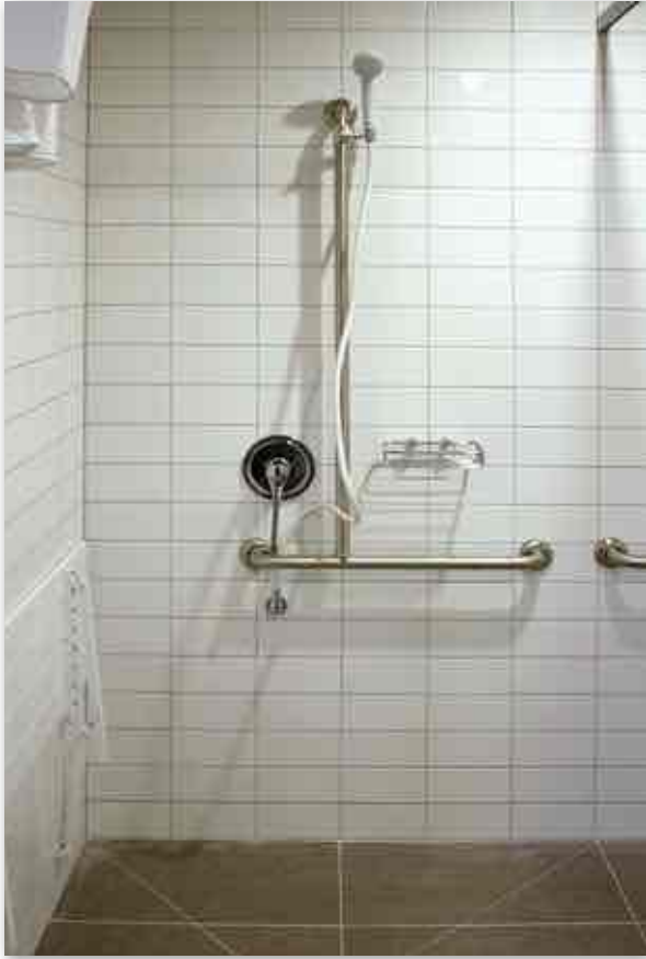
Example of an accessible shower facility Image courtesy of JMA Architects
