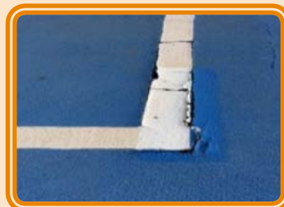
Asphalt damage due to oil based paint used
