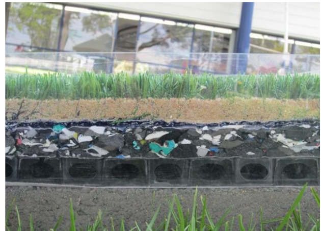
Photo 31: Example of horizontal drainage cell under shockpad (source: Wayne Stuart - City of Swan, WA)
