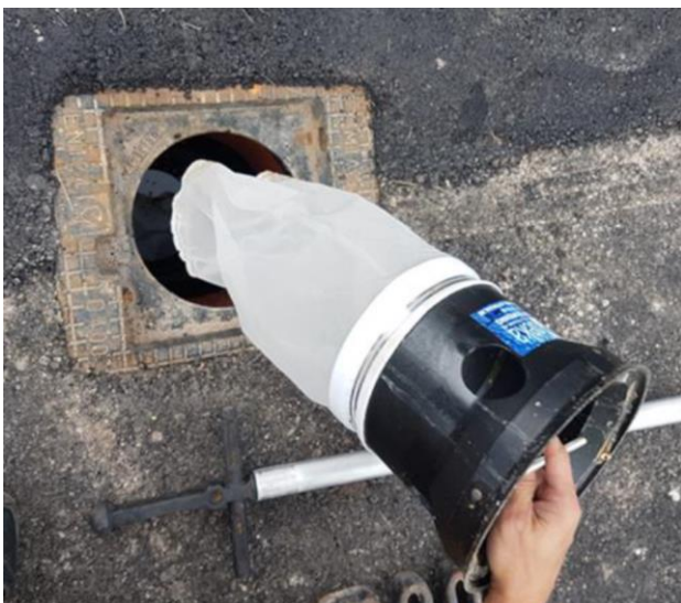
Photo 19: Containment strategy: Drains fitted with filter.
